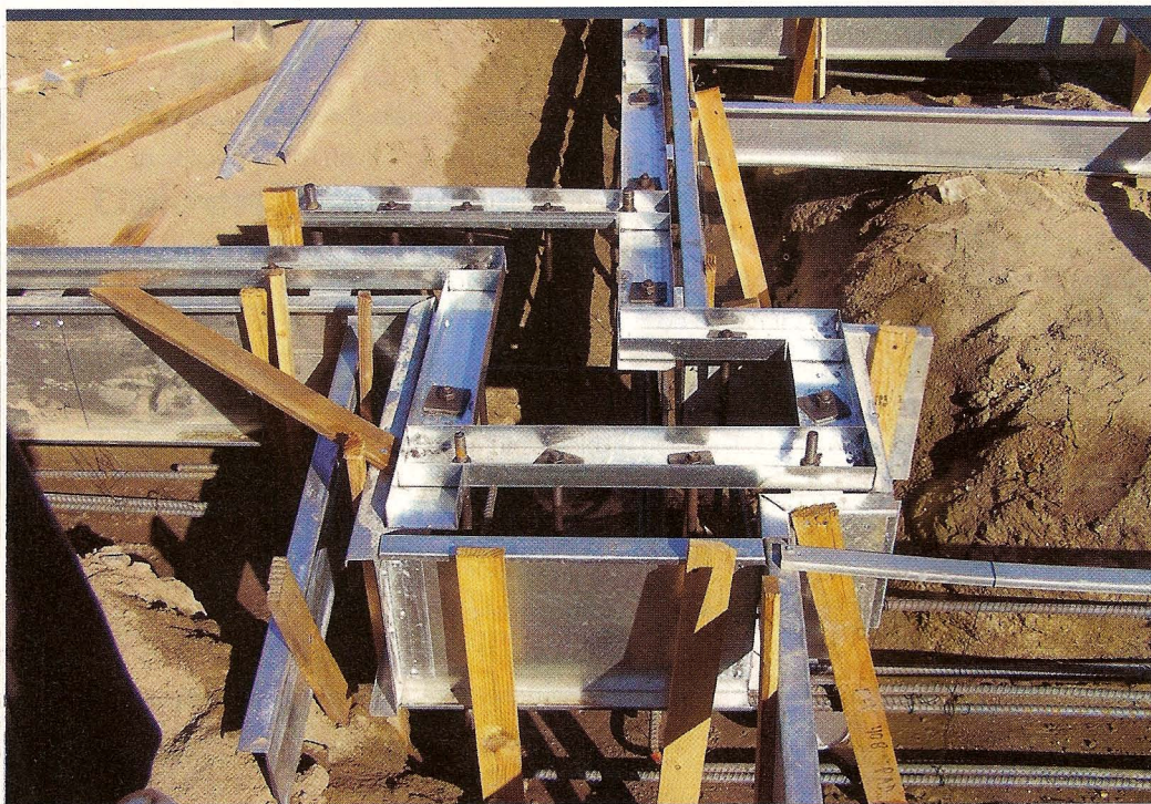
Setting the bottom plate in the slab for panelized walls is more difficult because codes restrict the use of epoxied anchor bolts. Fastening the bolts and setting the bottom plate prior to the pour allows the bolts and bottom track to be wet set in the concrete.
