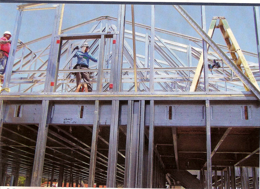
Balloon framing the first floor allows the steel framer to hang a ledger and install the second-floor joists more quickly. The floor diaphragm is sandwiched between the top plate of the first-floor wall and the bottom plate of the second-floor wall.
